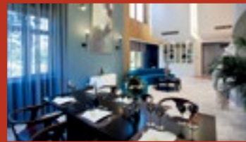
The 4 sets of GSHPs keep the indoor temperature within the range of 22-25°C. The blue film solar water heating system is equipped with 2 heat-collecting plates and a 200 L water tank.
